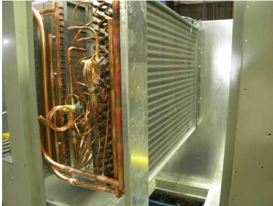
Figure 65. Evaporator and reheat coil
