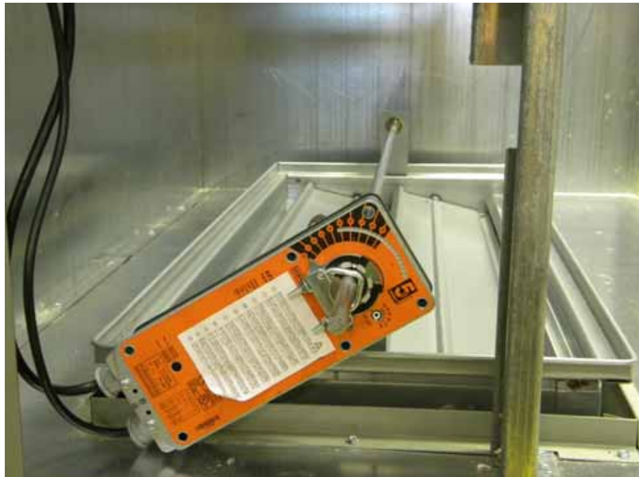
Figure 70. Return air damper
