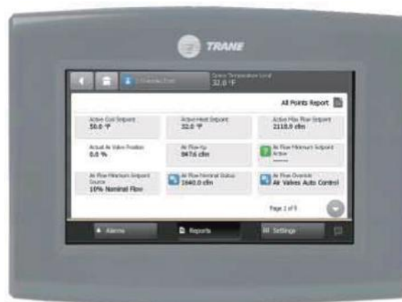
Figure 6 – TD7 operator interface
